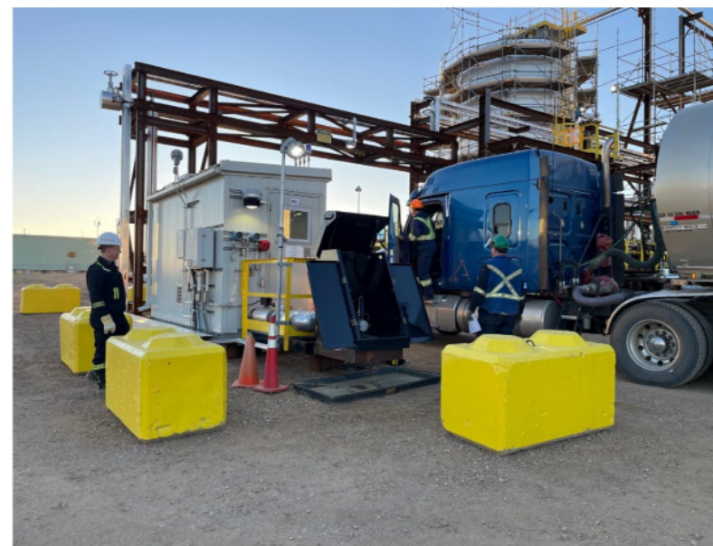
Truck Rack Commissioned in October 2022
