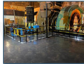
1 OF 4 UNDERGROUND WINDER CHAMBERS
