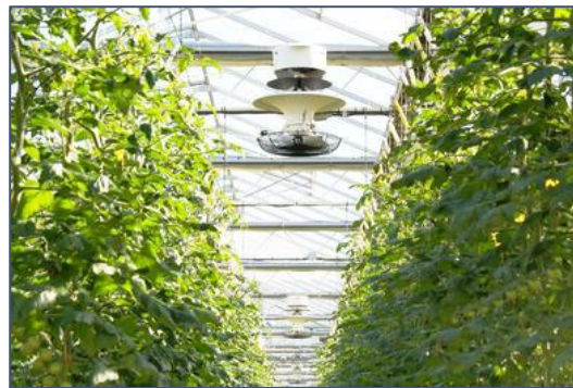
Ventilation cooling system
